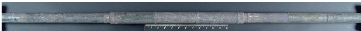
Figure 12. Section of samples removed from Äänevoima FB steam test loop during May 2017 annual shutdown
